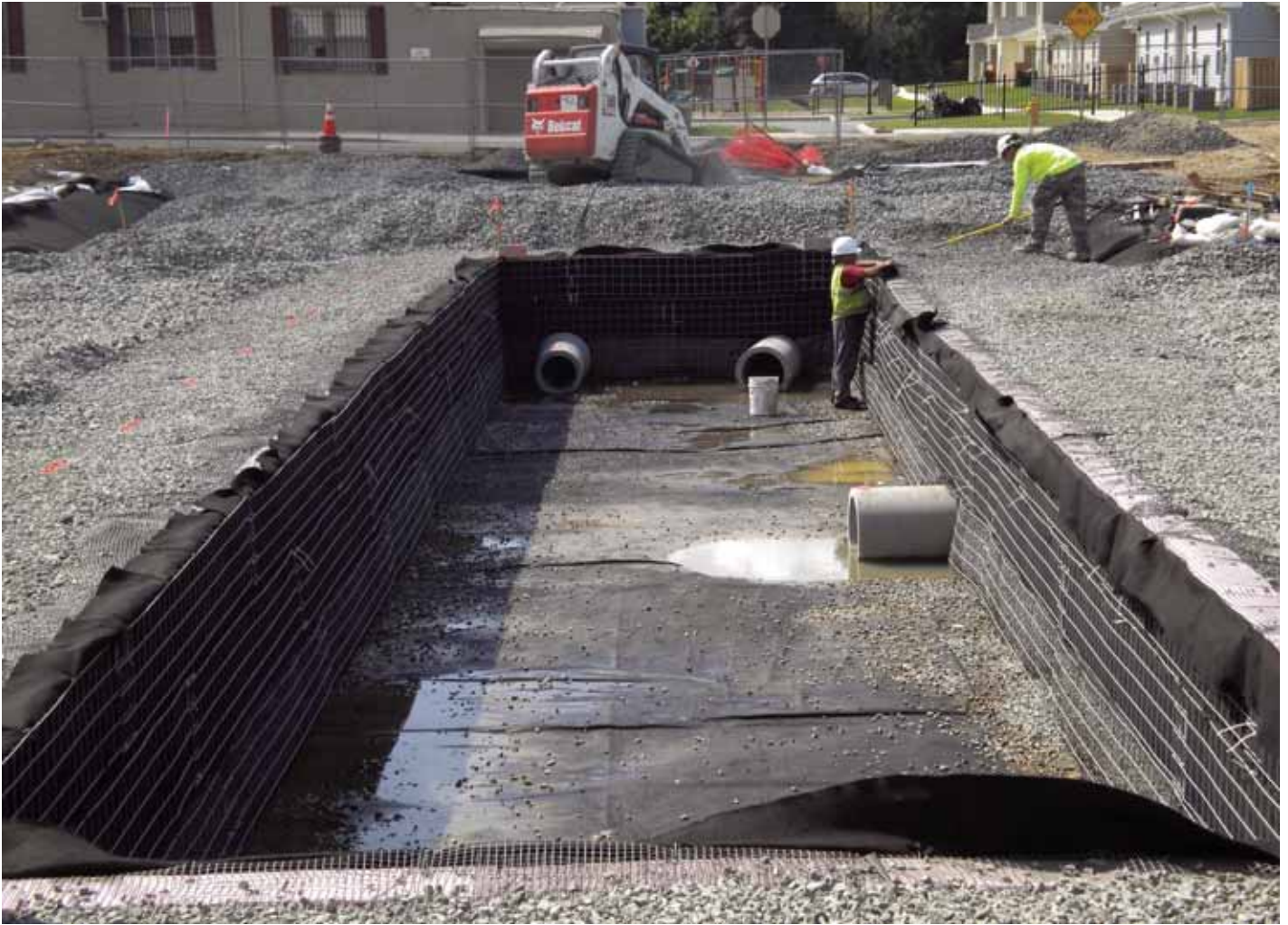
Stone walls are constructed around the perimeter of the lined excavation over the geomembrane and stabilized with geosynthetic reinforcement at tightly spaced lifts.
